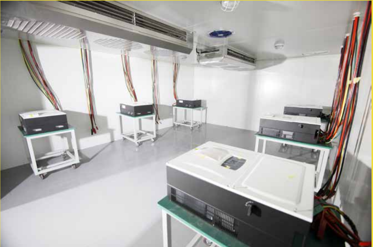
Zeversolar testing chamber
